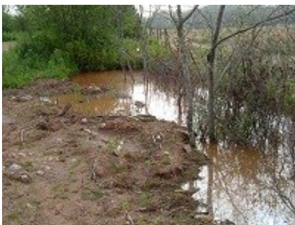
“The track bed in one area is causing flooding.”
