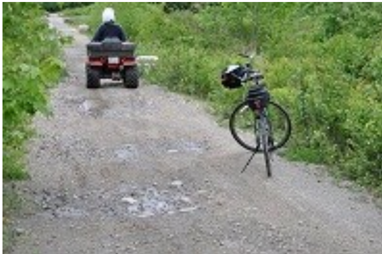
Motorized trails cost 3-4 times as much as Active Transportation trails to maintain. Note damage starting to show on this trail.
